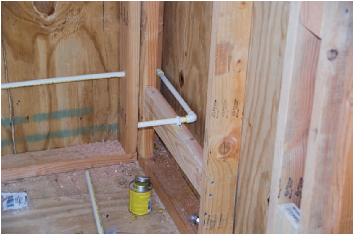
Cold Pipe for Toilet
