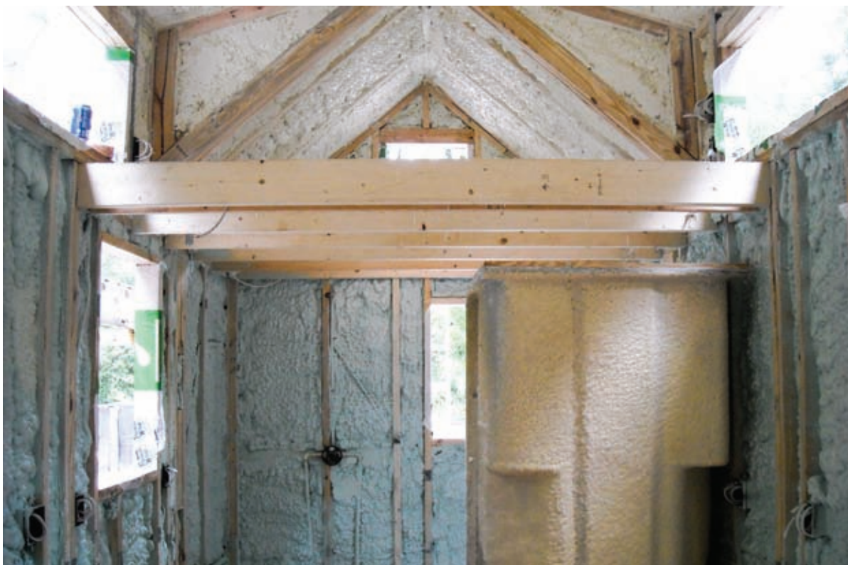
Closed Cell Spray Foam
