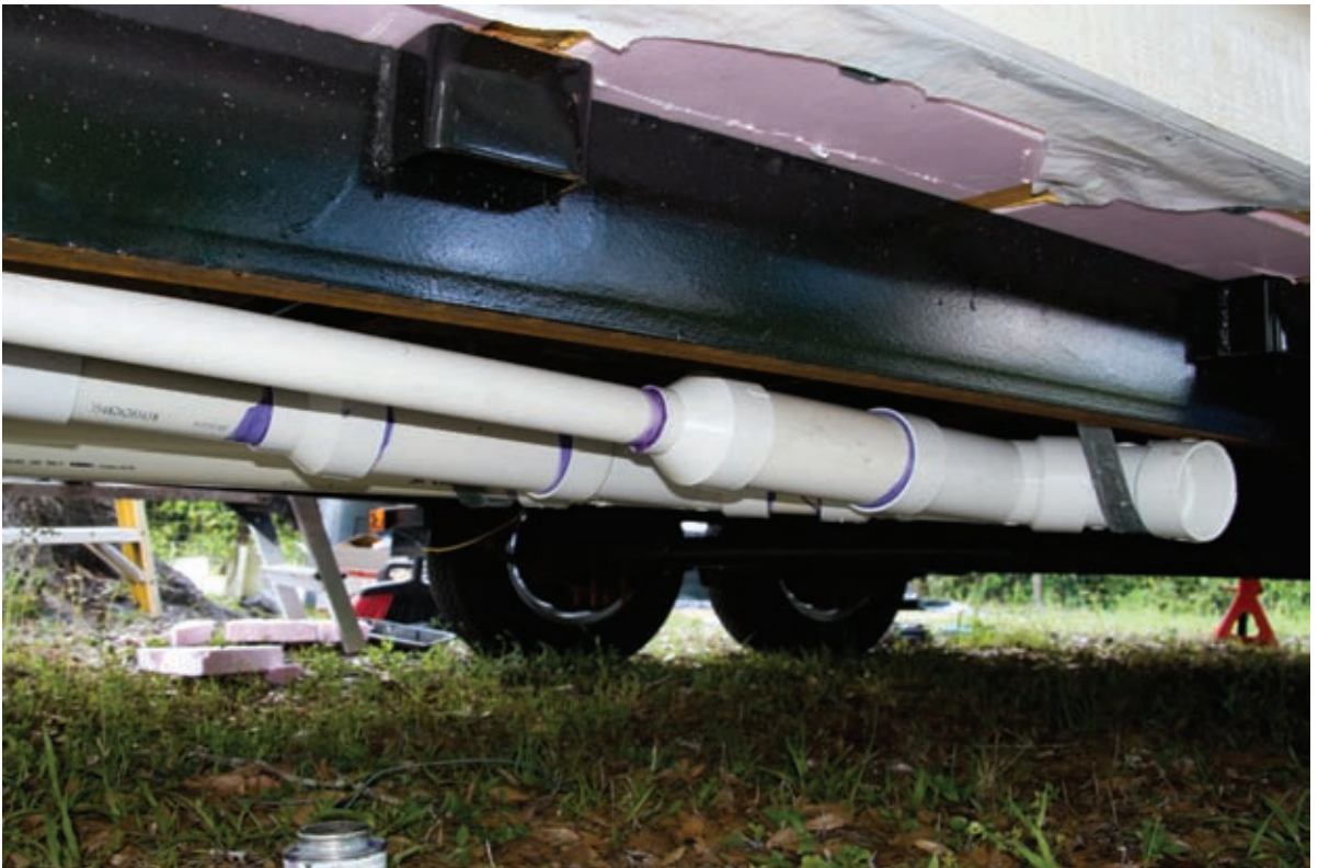
Drainage Pipes Under Trailer
