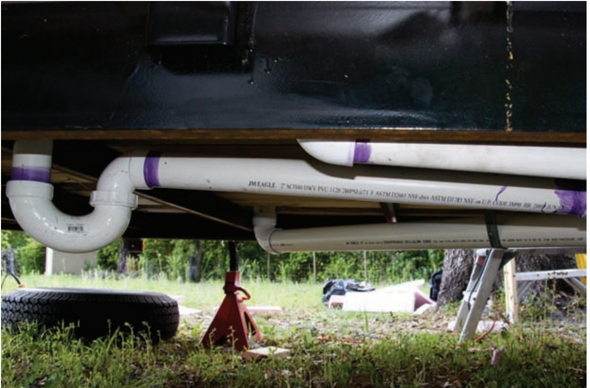
Drainage Pipes Under Trailer
