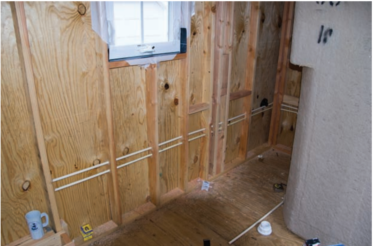
Hot and Cold Pipes for Kitchen Sink
