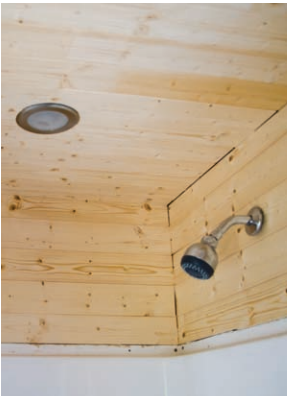
Untrimmed Interior Siding Above Shower
