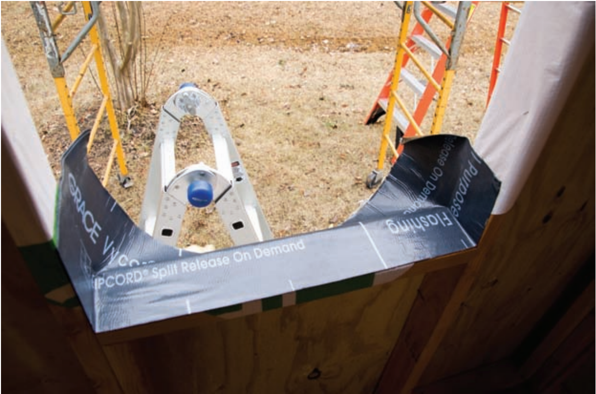
Flashing Partially Attached to Sill Plate
