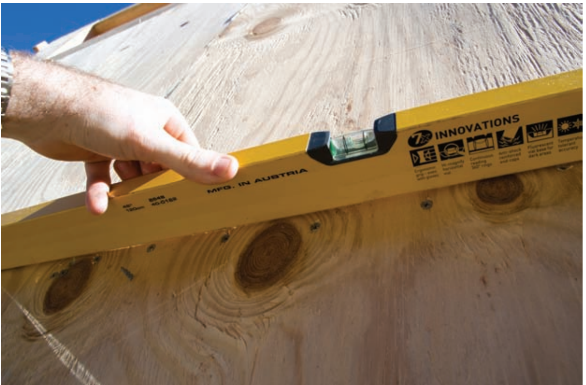
Wall No Longer Warped
