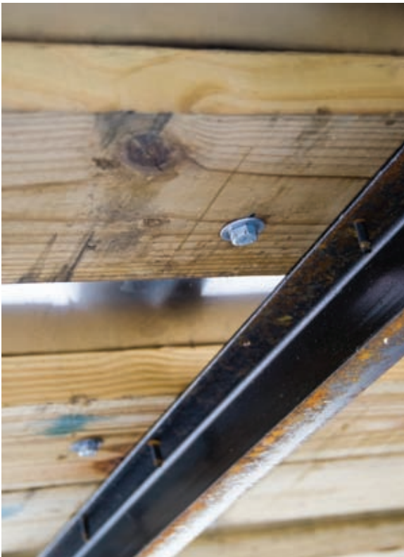
Lag Screws Under the Trailer
