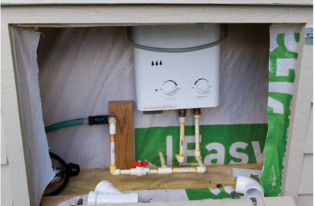
Hot Water Heater
