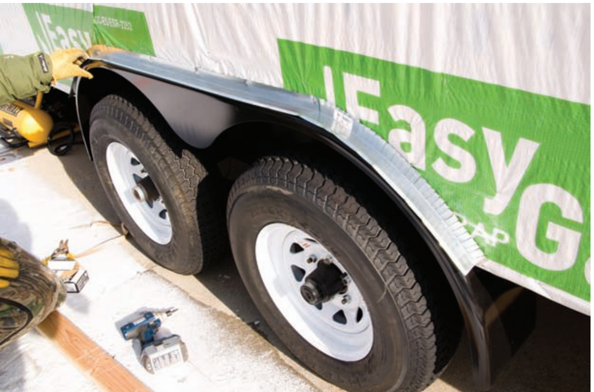
Flashing Over Wheel Well
