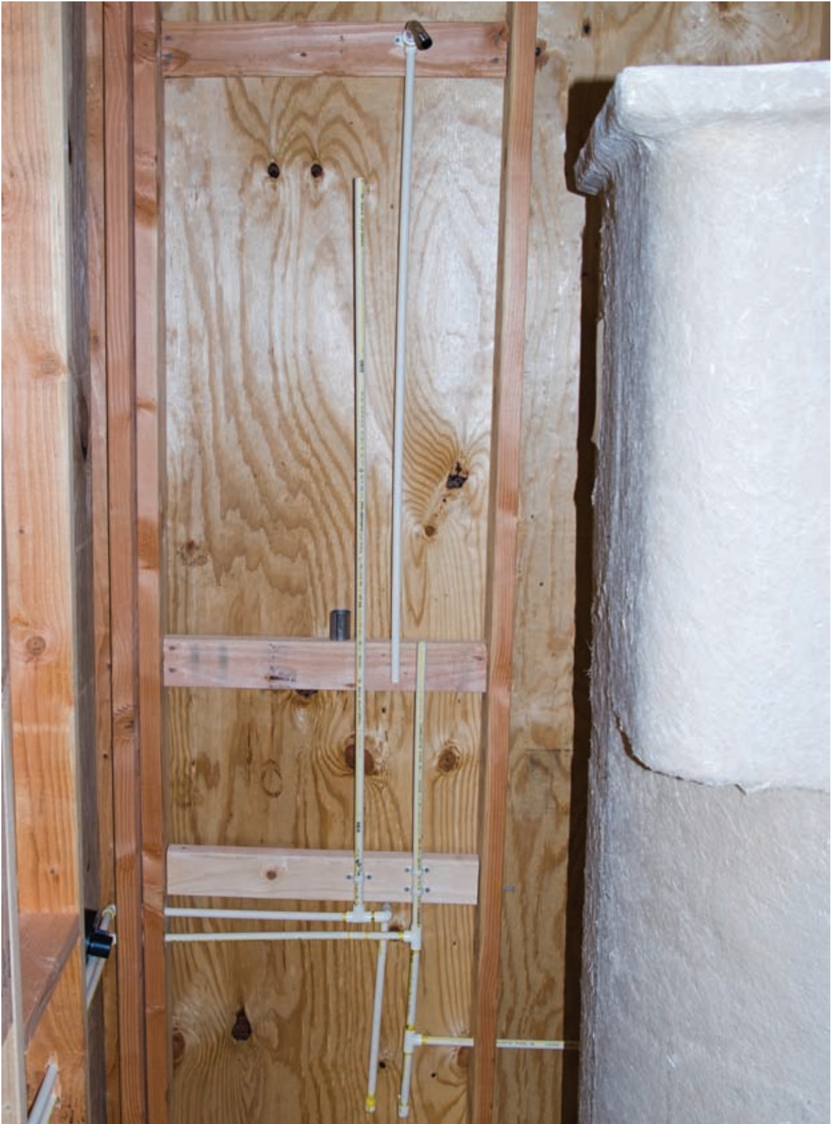
Supply Entry and Shower Hookup
