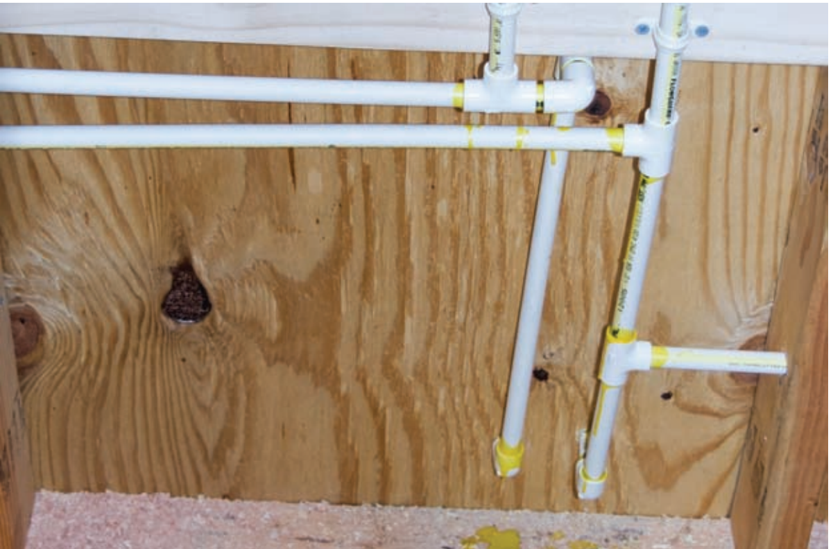
Supply Entry Into House
